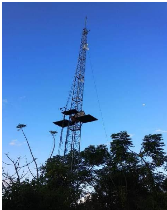
Figure 7: Wireless network tower on Bunaken Island.
