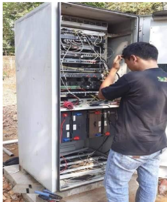
Figure 12: Outdoor Cable House at the center of AWI.NET.ID.
