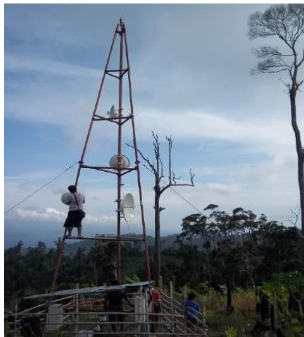
Figure 6: Wireless Network Tower in Sidangoli, West Halmahera.
